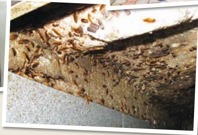
German Cockroaches have taken residence in this rubbish chute.
