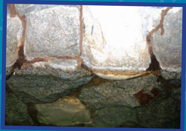
Worker termites built this mud tube to draw water from an in-door fish pond.
